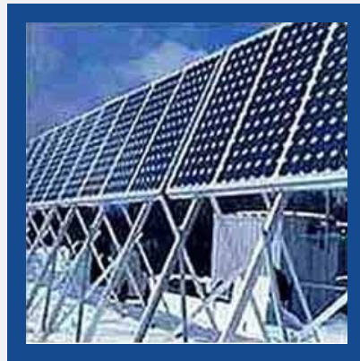
Solar Power Plant
